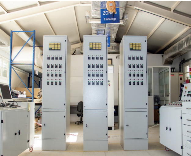
Project: Electrical Panels (Libya) Year: 2021
