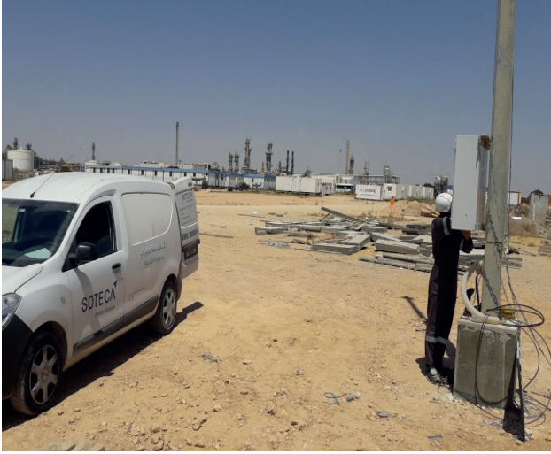
Project: Electrical Installation (Nakta - Tunisia) Year: 2014
