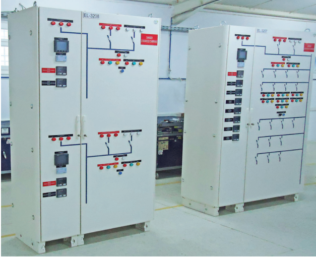
Project: Supply & installation of electrical distribution equipment (Sfax - Tunisia) Year: 2008
