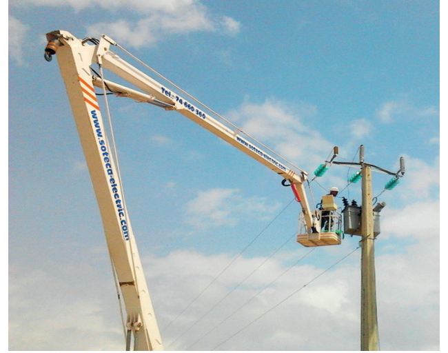
Project: Transformer Station (Kerkennah, Sfax - Tunisia) Year: 2017
