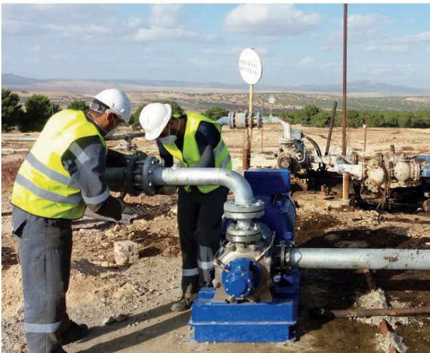
Project: Electrical works in an oil pumping station (Douleb - Tunisia) Year: 2021
