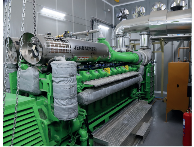
Project: Cogeneration (Sfax - Tunisia) Client: STPA
