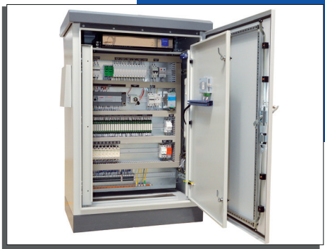
Crossroads light control cabinet
