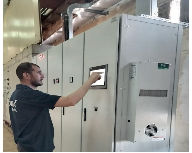
Project: Replacement of wired-logic control panels with automated-logic control panels (Tunis - Tunisia) Client: RNTA
