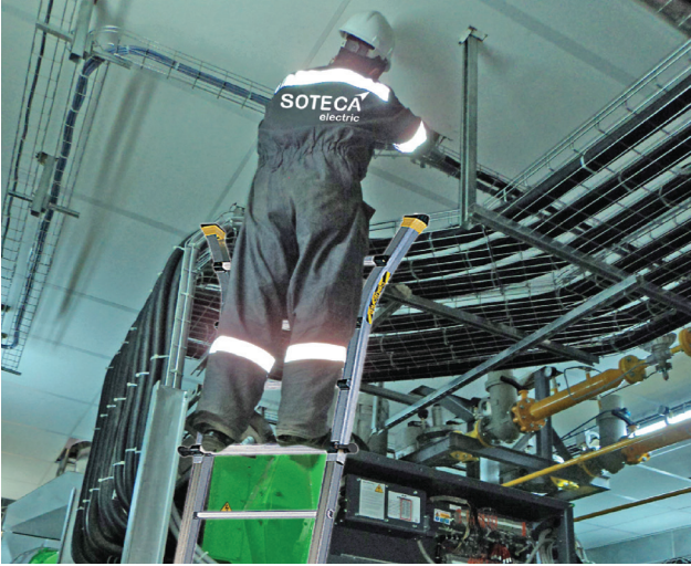
Project: Cogeneration (Sousse - Tunisia)
