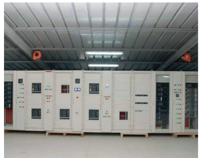
Project: Export of Electrical Panels for the Felix-Guyon Hospital Center ( Ile de la reunion - France ) Client: Cegelec - Vinci
