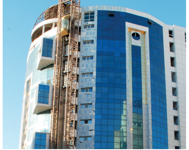
Project: Iheb Center (Sfax - Tunisia) Client: Al Faraana Company
