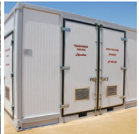
Project: Shelter for electrical transformation and distribution equipped with panels in medium and low voltage (Libya) Client: GECOL
