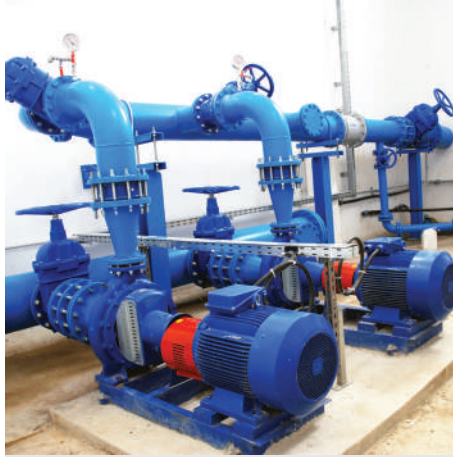
Project: Recovery Pumping Station (Dokhane-Tunisia) Client: SONEDE
